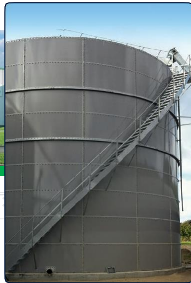
TANKS AND SILOS DEPÓSITOS
